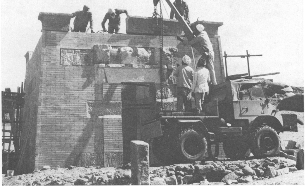
1. The last stage of re-erection. An embankment has been made, up which the small mobile crane has been driven so that the cornice block can be hoisted to the required height
